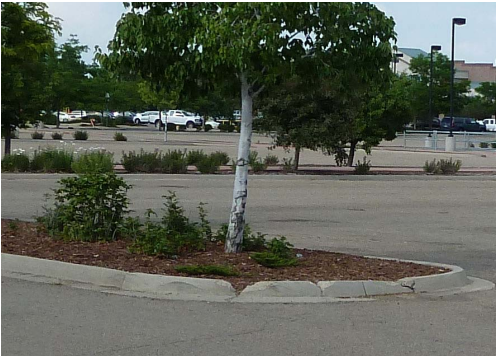
Various portions of damaged curb and gutter were found
