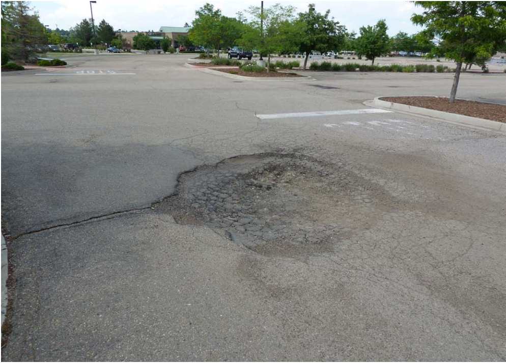
The parking had cracks and potholes in places
