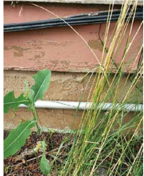
Foundation cracking viewed from the exterior.
