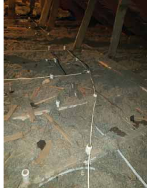
Extensive knob and tube wiring in the attic.
