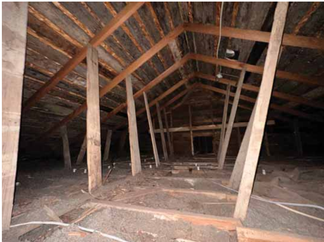
Main gable roof framing with access hatch to front porch roof framing.
