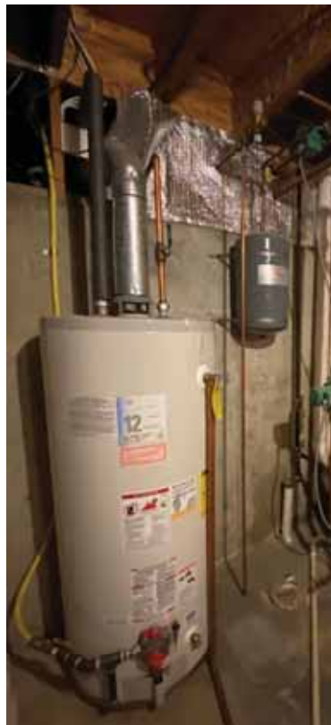
Water heater & side-arm
