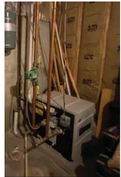
High efficiency boiler
