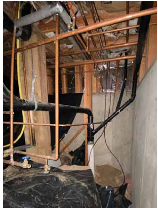
Copper water supply and plastic waste lines
