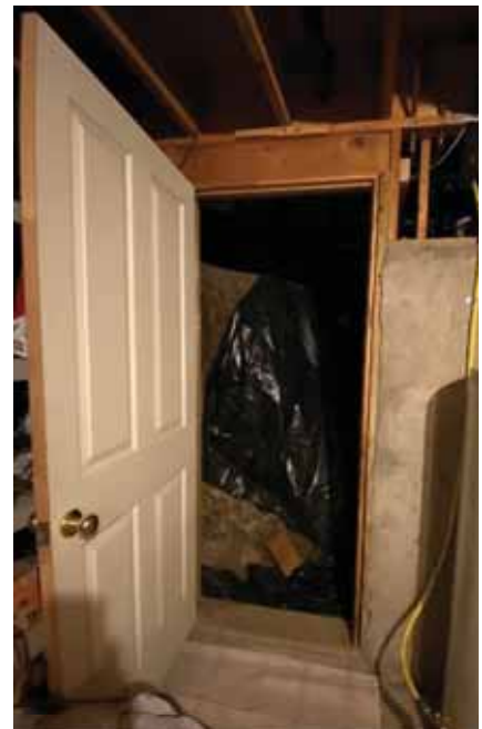
Separation between basement & crawlspace in mechanical room. Poured concrete wall with cripple wall above on the right
