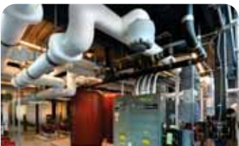
McKinstry developed the South Landing all electric district heating/cooling system, which is 4x more efficient than a code based system.
