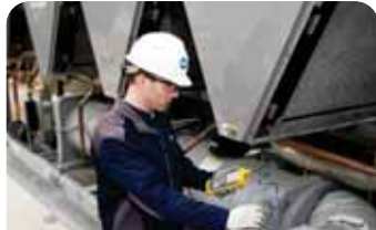
McKinstry recently reduced one client's carbon footprint by 18%, just through Advanced Building Optimization!
