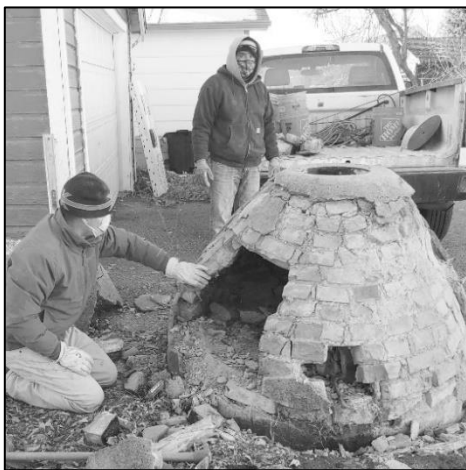
In November 2020, Olde English Masonry carefully took apart the ash pit shown on page 1. Moving it while intact proved to be too difficult.
