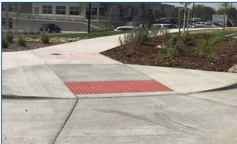
Curb ramps are generally consistent at intersections, which improves the overall accessibility for people walking or using mobility devices such as wheel chairs.
